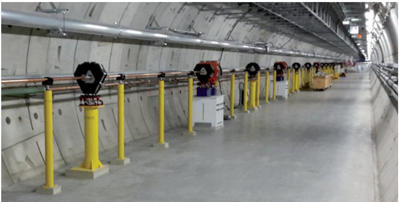
Fig. 14 - Agilent In-line Ion pumps integrated into a transport beam-line at X-FEL/Desy.
