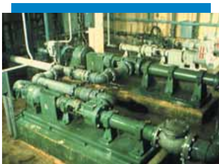
These Moyno pumps were installed in the early 1960s to feed sludge to a belt filter press for dewatering. Moyno pumps deliver a steady, consistent flow of material to any dewatering device, which is a critical aspect of dewatering efficiency. With a rugged drive train design and advanced rotor/stator technology, Moyno pumps deliver years of trouble-free performance.
