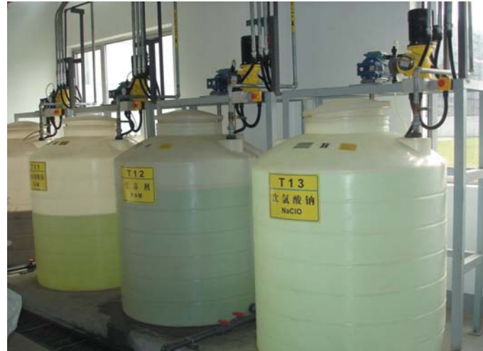
污水厂加药装置 The sewage plant dosing device
