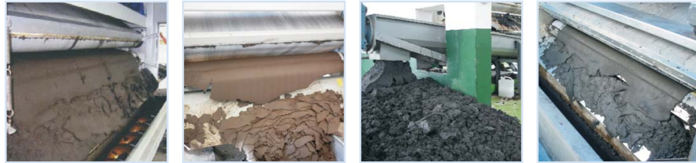
市政污水 Municipal Sewage Treatment Plant
