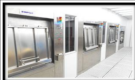
Multiple DI Water Washing - Unloading
